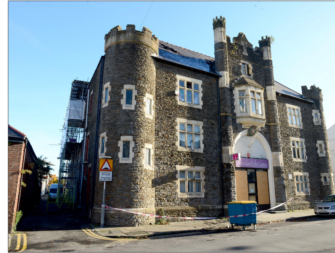
WORK: The fire damaged Abundant Life Centre in Lower Dock Street, Newport, after the 2016 fire
