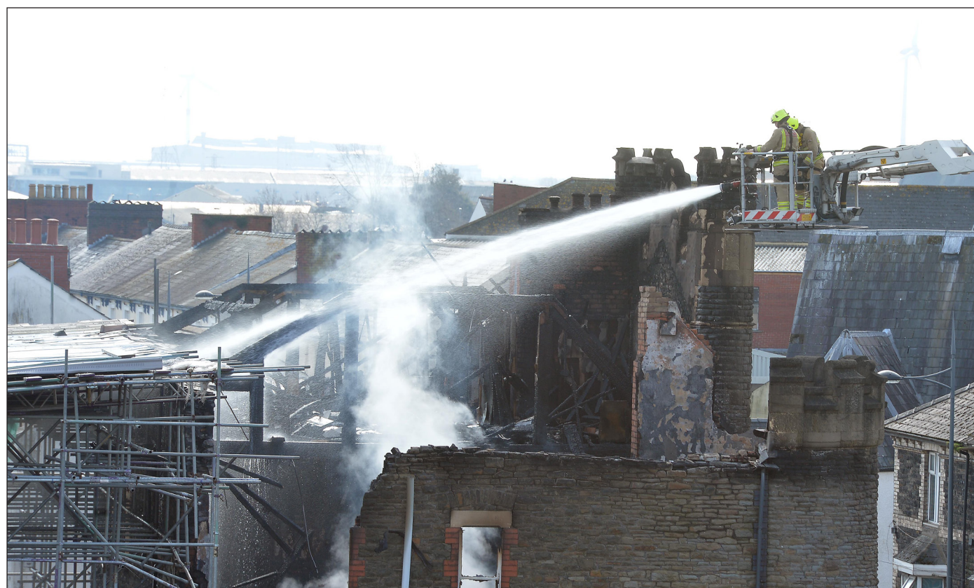
DAMAGE: Firefighters damping down the fire at the Abundant Life Centre in Lower Dock Street, Newport. Picture: www.christinsleyphotography.co.uk.
